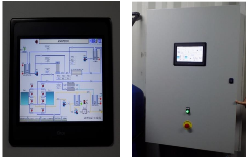
Figure 13. electrical panel photos
